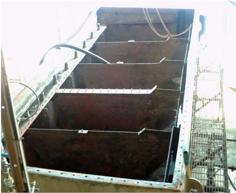
The photo shows the top cover plate removed and the IGF Cleaned by Enviro-Tech Systems Personnel
