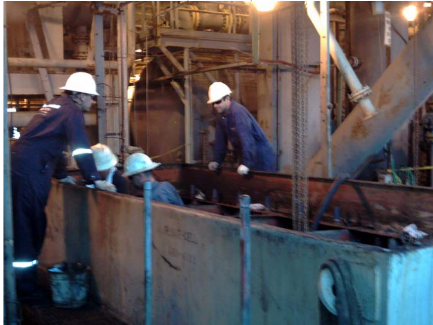
The photograph shows the Enviro-Tech team working to install new internal parts.
